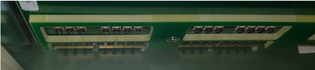
Xlink boards INCORRECTLY below mating connectors
