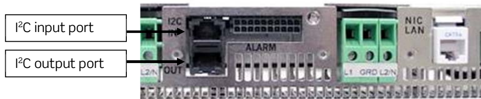
Figure 19 - I 2 C Communication Ports
